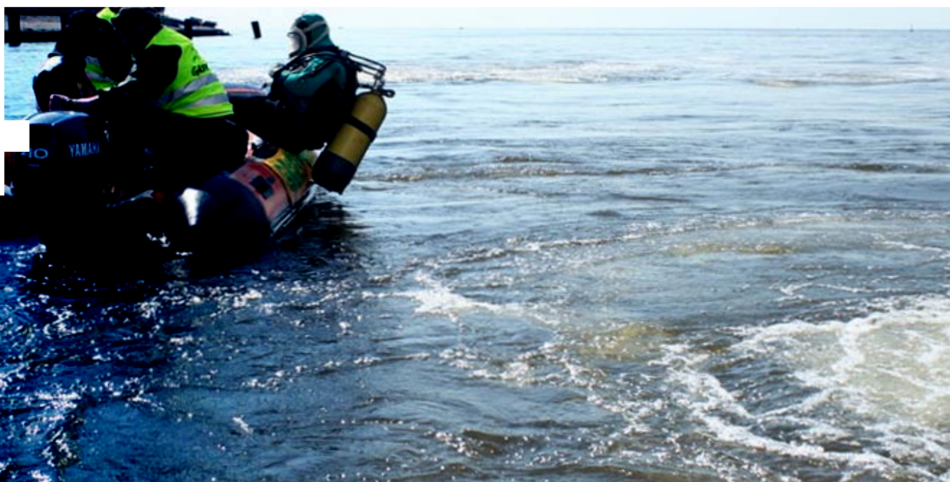
Underwater effluent dispersing pipe of Central WWTP, located at Nevskaya Guba, Gulf of Finland, St-Petersburg, Russia, 2007. © Greenpeace
